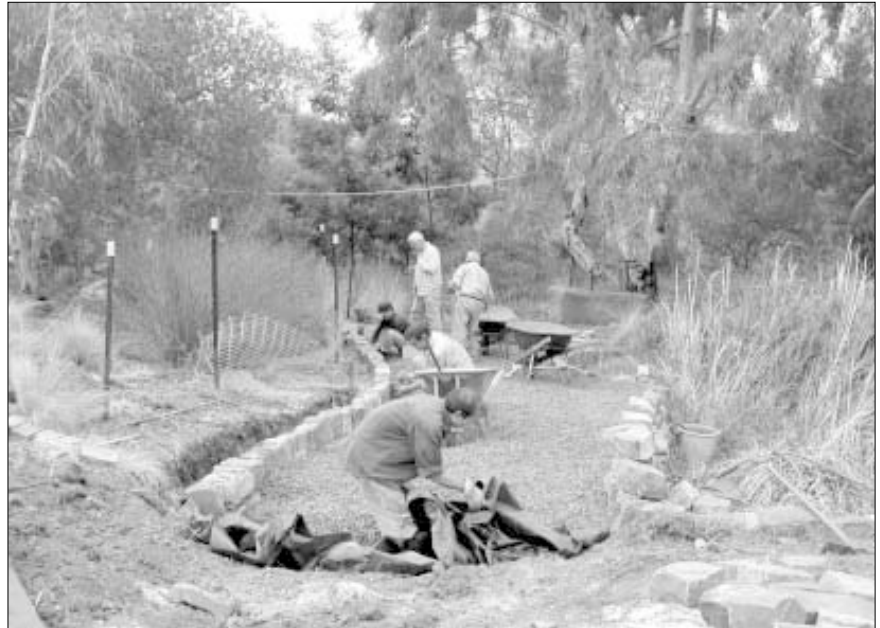
CERES Green Technology workshop staff and volunteers reconstruct the reedbeds for the new and improved system that recycles water from the cafe and toilets.
