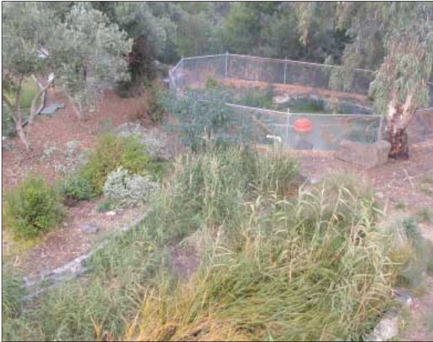
The improved reedbed filtration area and the new holding pond, the last stop for the wastewater before it is pumped out and used to irrigate the Village Green.
